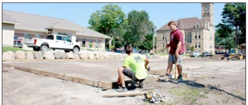
Work has begun on a new residential duplex being built on the former First Baptist Church property in downtown Grundy Center. (Michaela Kendall/The Grundy Register photo)
